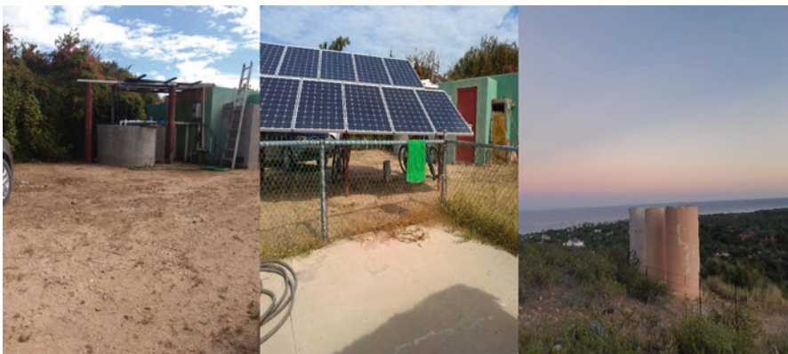
Fig. 28.2 Promotora Pelicano SA de CV's hydraulic infrastructure
